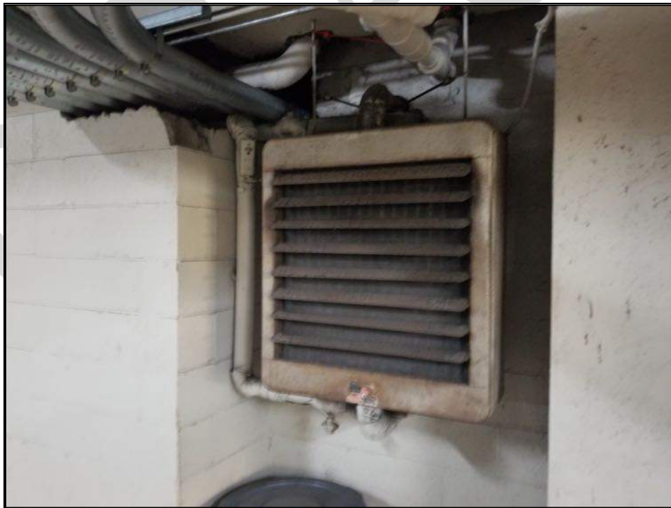
TYPICAL GARAGE UNIT HEATER.
