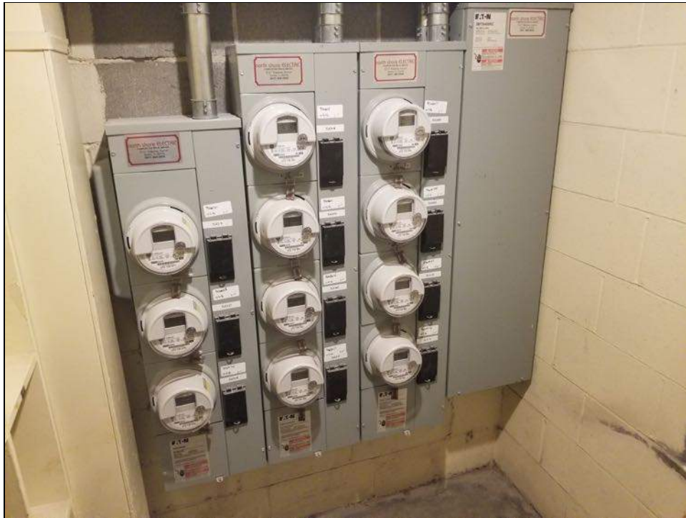
TYPICAL FLOOR ELECTRICAL CLOSET
