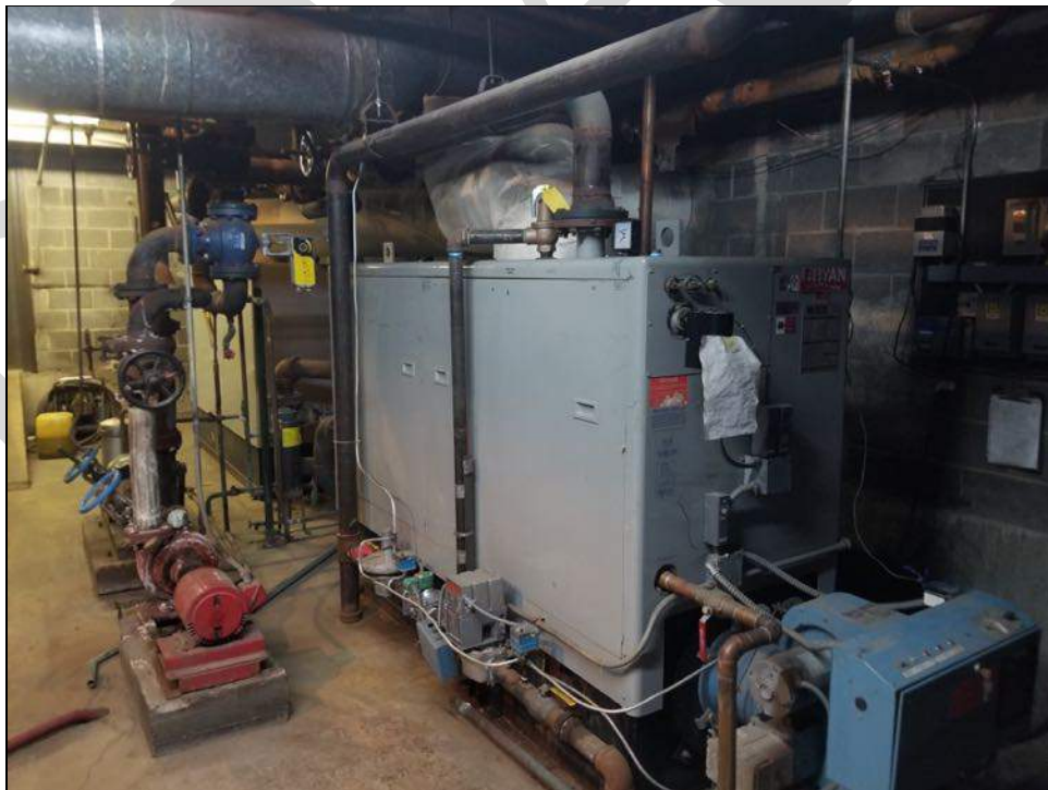
BUILDING HOT WATER BOILERS.
