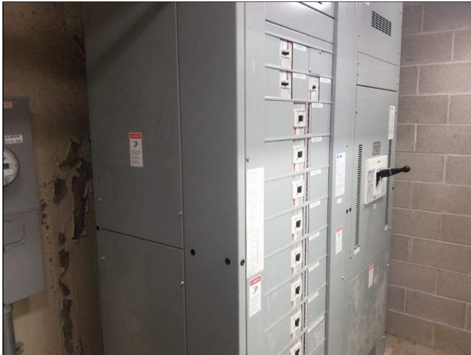
MAIN ELECTRICAL SERVICE
