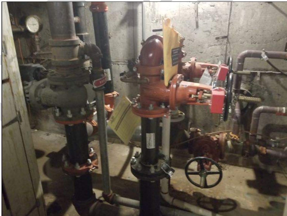
FIRE SPRINKLER PUMP.
