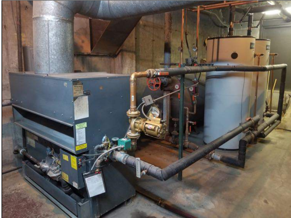
DOMESTIC HOT WATER BOILER AND HOLDING TANKS
